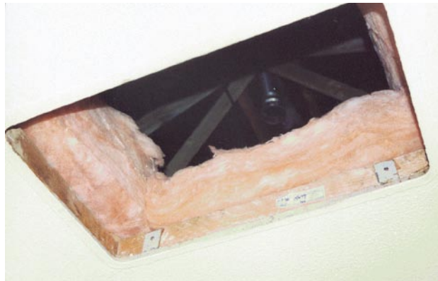
▲ A loft access hatch, showing the loft insulation after refurbishment, showing that the insulation fills the loft space and that there is no significant thermal bridging at the loft hatch
