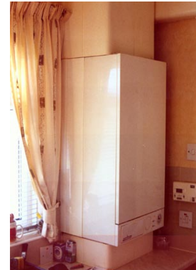
▲ The condensing boiler in one house within the scheme
