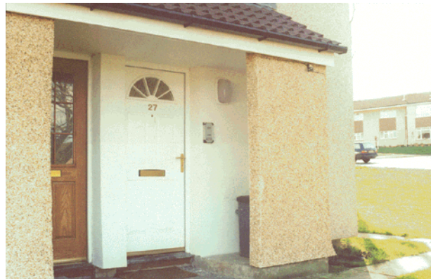
▲ The entrance to one of the houses, showing the external wall insulation taken almost to ground level. External insulation is also applied between the doors of the two adjacent dwellings
