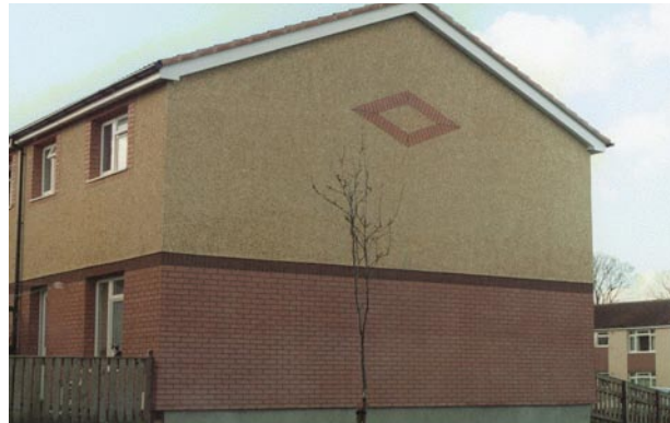
▲ An image of a gable wall, showing how it was not always practicable to extend the external wall insulation down to ground level. In this example, there is a gap of at least 300 mm between the ground level and the bottom of the external wall insulation
