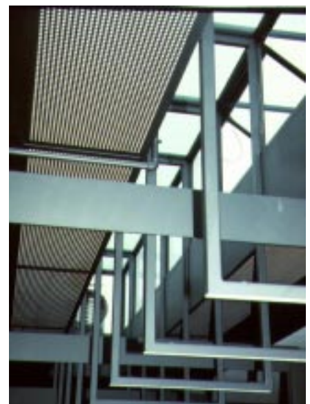
Figure 5: Location of Extract Fan and Open Roof Light
