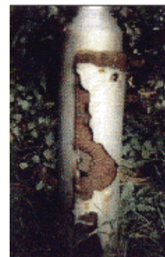
Corrosion of Steel Pole (A & M)
