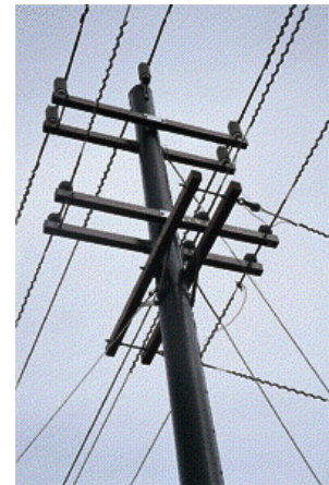
Utility pole supporting electricity cables (Shakespeare)
