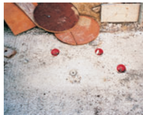
Figure 3: Floating cups grouped at edge of pour. One has already been pulled out.
