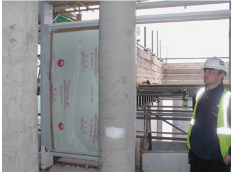
Figure 1: The improved finish from the use of self-compacting concrete for vertical elements
